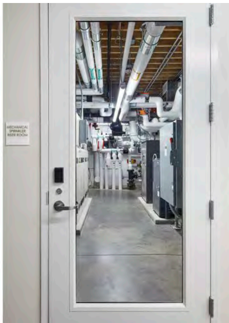
Above: Image of mechanical room, showing some systems
